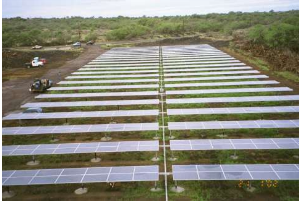
250 kW Solar Array Mauna Lani Resort in Hawaii Source: http://www.thesolarplan.com/articles/mlb3-fromlift.jpg
